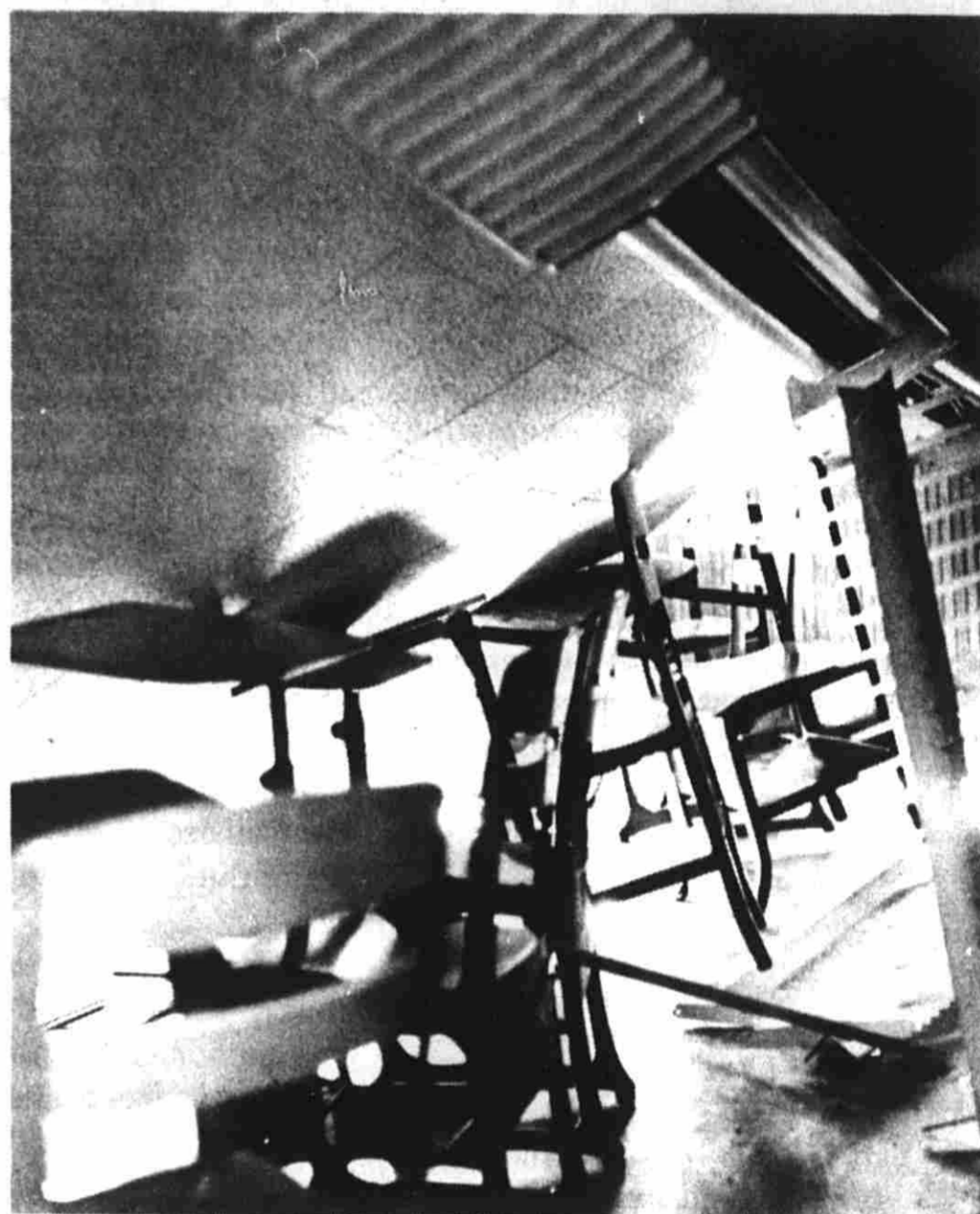
OUCH—Students fared better than these desks and escaped injury Nov. 20 when the ceiling in Van Raalte 206 collapsed.
